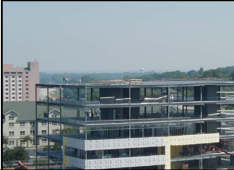
The 5 story building at 1241 John Q Hammons has reached its full height. The exterior walls are being prepared for the limestone panels.
